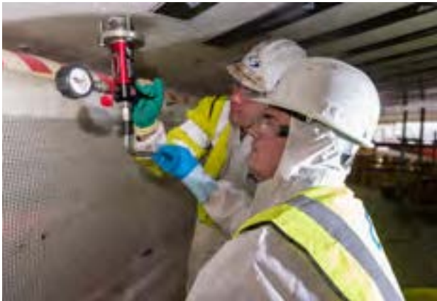
Pull-off test to test cohesive strength of concrete substrate after surface preparation
