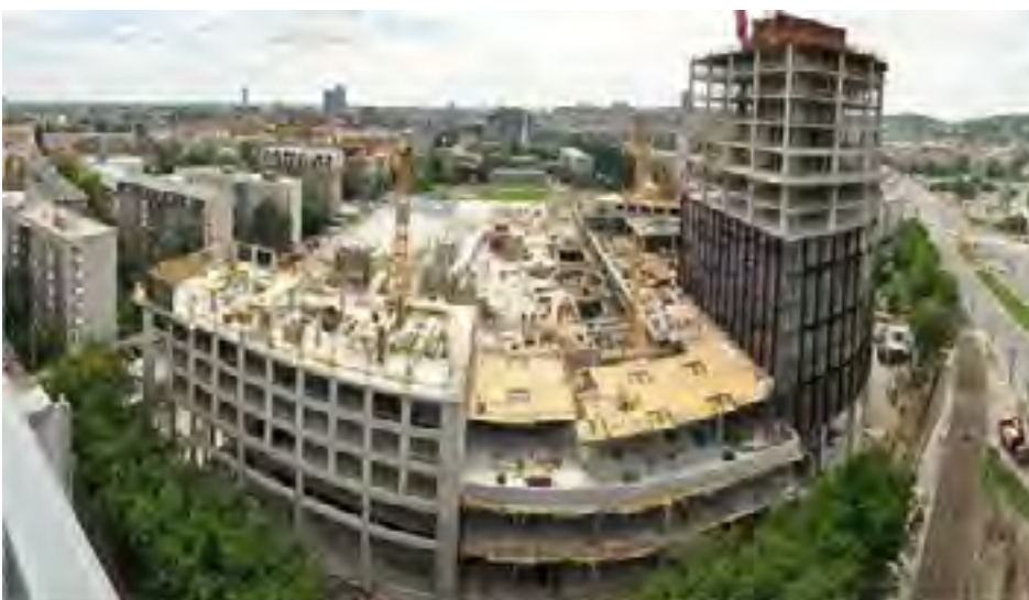
During construction time: The roof of the shopping center will offer a 6,000 m 2 natural setting and ample opportunities for an entire family to relax.
