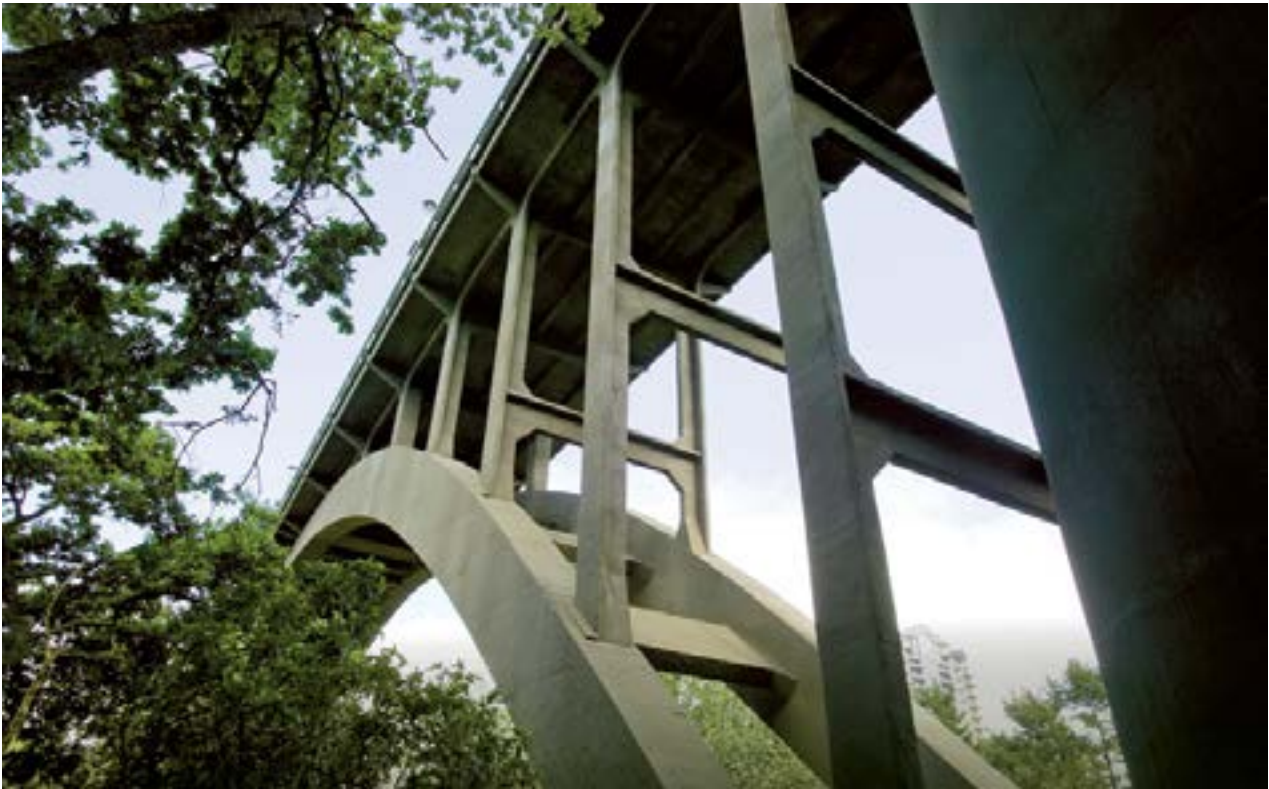
Auckland's Grafton Bridge, the world's largest single span reinforced concrete arch bridge when constructed in 1910, has continued its history of innovation by using Sika CarboShear technology in its 2010 strengthening. Sika CarboDur® plates provide flexural and shear strengthening
